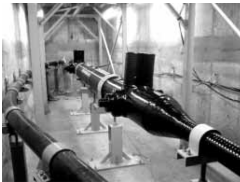
Photo 3. HTS Cable-to-cable Joint in Underground Vault
