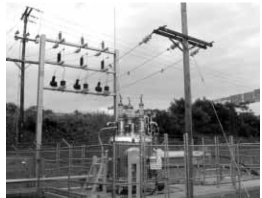
Photo 5. HTS Cable System Connected to Overhead Power Lines
