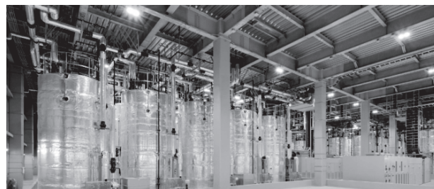
1st floor: Installed PCSs, tanks, and pumps
