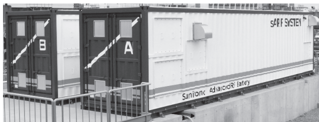
Photo 2. Exterior of container system
