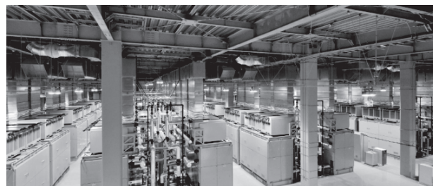
2nd floor: Installed battery cubicles and BMS
