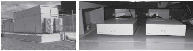
PCS enclosure (on the left), installation status in the PCS (on the right)
