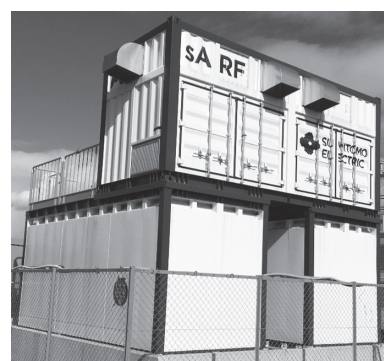
Photo 2. Example of container-type 250 kW × 3 h RFB system
