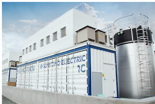
Fig. Redox flow battery (RFB) system installed in California
