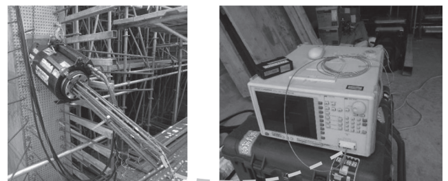
Photo 4. Example of measurement for internal cable
