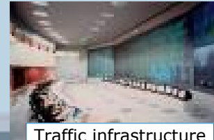
Traffic infrastructure control
