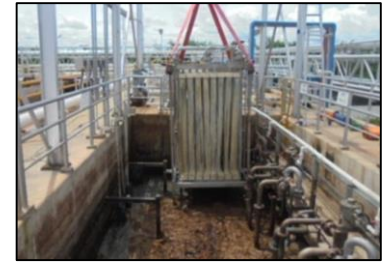
Textile dyeing plant in Thailand Respond to the tightening of regulations on the quality of water to be discharged.
