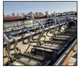
Sewage treatment facility in China Improve the quality of the water in the river to which water is discharged from the facility.
