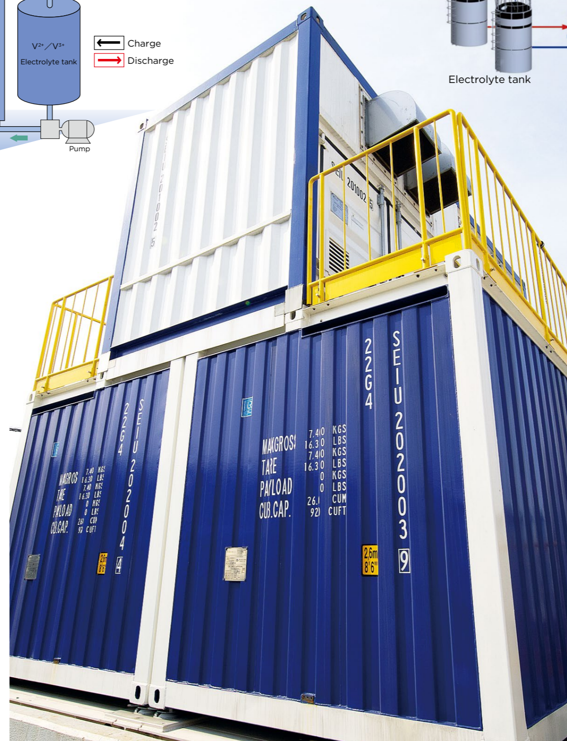
A redox flow battery consists of three devices: positive and negative electrolyte tanks installed on the first floor and cell stacks with electrolytic baths installed on the second floor.
