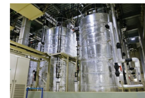
Electrolyte tanks in the building
