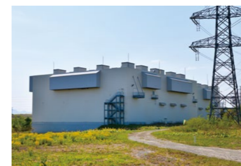
Energy storage battery building
