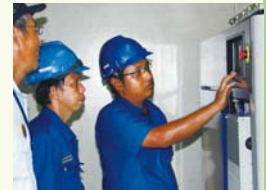
Reduction of the revolution speed of the paint feed pump by installing an inverter
