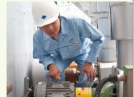
Replacement of a pump in the effluent treatment plant with a high efficiency pump
