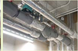
Thermal insulation of steam pipes
