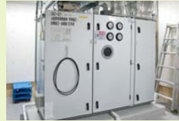
Intermittent stop of the outside air treating air conditioner
