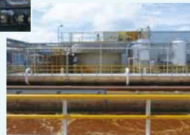
Wastewater treatment system installed in the Thailand Plant
