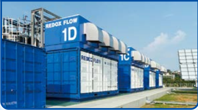
Redox Flow Battery
