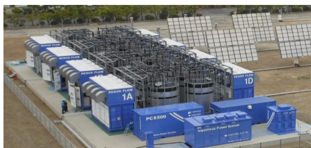
Redox Flow Battery
