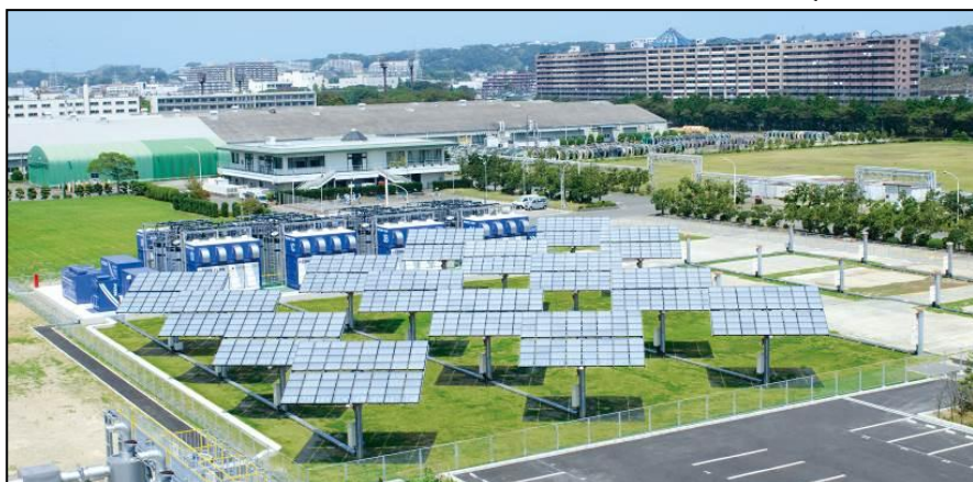
SEI Yokohama Works redox flow battery & CPV system
