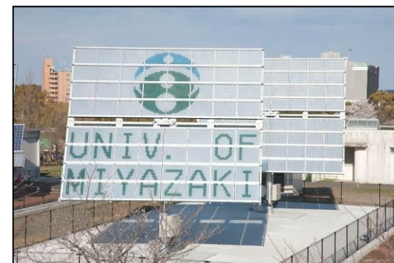
CPV installed at the University of Miyazaki
