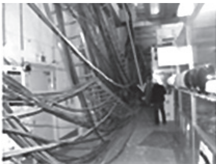
Photo 1. Fallen Cable Racks
