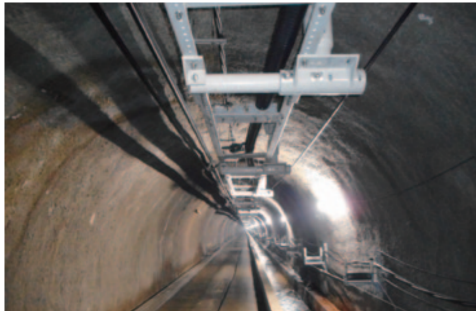
After being pulled into the tunnel, the cable is placed on supports mounted on the ceiling.
