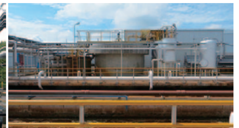
Wastewater treatment system installed in the Thailand Plant
