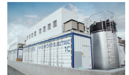
2-MW/8-MWh Redox Flow Battery in California, USA
