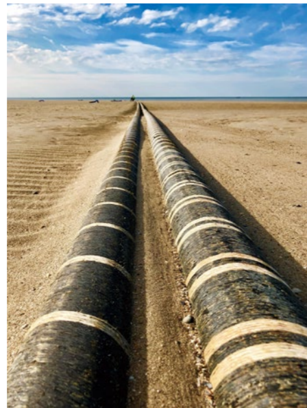
Nemo Link interconnector cables to be installed between UK and Belgium (before cable burial)
