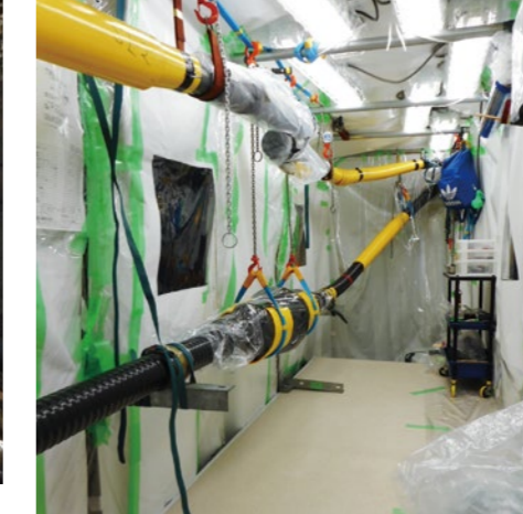
Cable connection room: Workers made efforts to implement dustproof measures in the severe environment.
