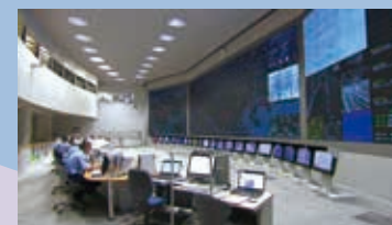
Traffic control system
