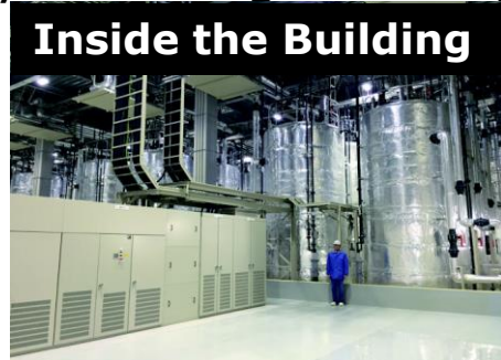
Hokkaido Electric RF Battery Building
