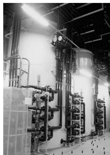
Photo 4. Instantaneous Voltage Sag Compensation 3 MW System (Electrolyte Tanks)
