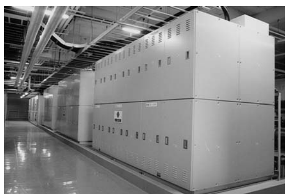
Photo 3. Instantaneous Voltage Sag Compensation 3 MW System (Battery Cubicles)
