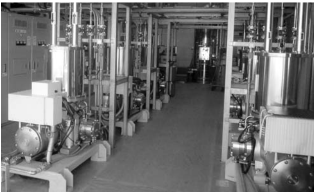
Photo 5. Cooling System after Installation
