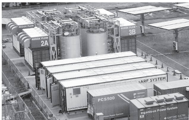
Photo 1. RFB system at Yokohama Works
