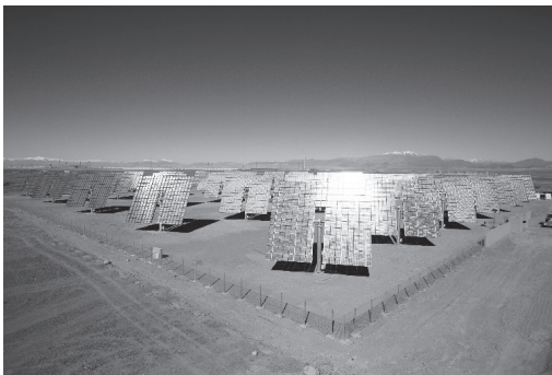
Photo 2. Megawatt-Class CPV System Overview in Ouarzazate
