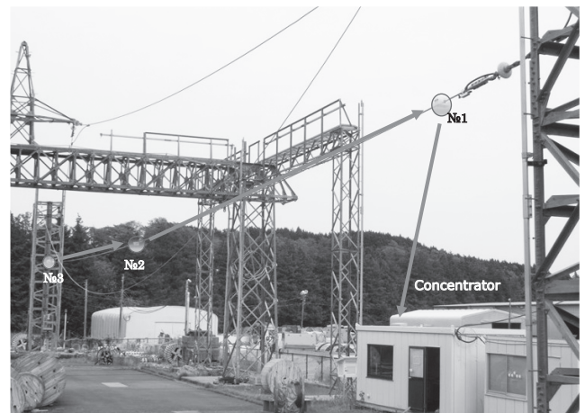
Photo 6. Terminal operation test under live condition
