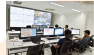
Traffic control systems These systems collect and analyze a wide range of transport information and use it to control traffic lights and provide transport information, enabling a safe and smooth flow of traffic.
