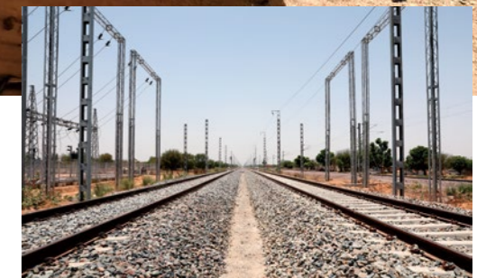
Orderly rows of poles are erected alongside rails before installing contact wires on the railroad
