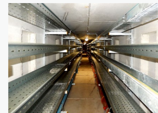
MCF-equipped underground tunnel in city of L'Aquila
