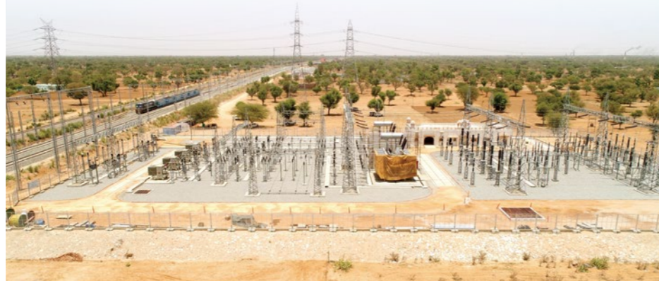
Substation built in a desert beside a railroad; To ensure stable power supply, substations are built equidistantly within a total distance of 1,500 km.
