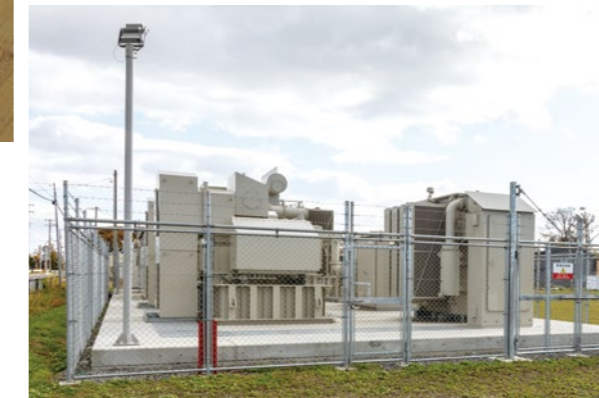
Grid connection switching station
