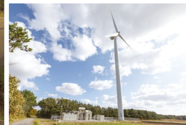
A completed wind turbine and an adjacent substation
