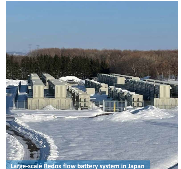
Large-scale Redox flow battery system in Japan
