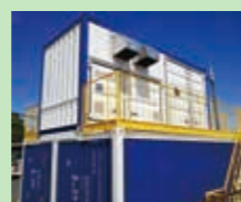
Redox flow batteries
