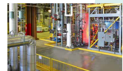
Plant in NY, U.S.A. with recycling system
